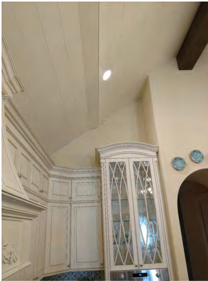
Damaged wood ceiling
