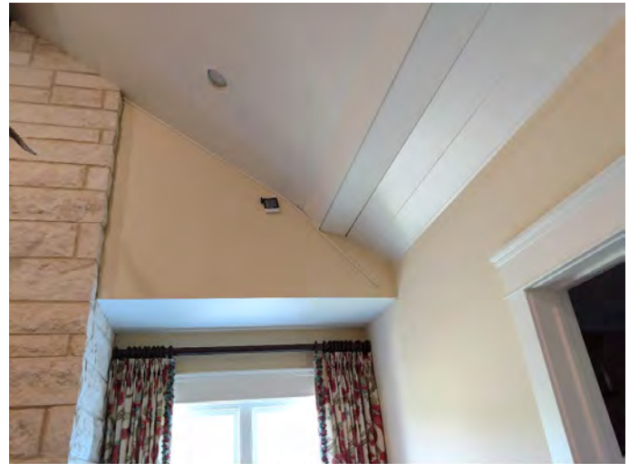
Damaged wood ceiling
