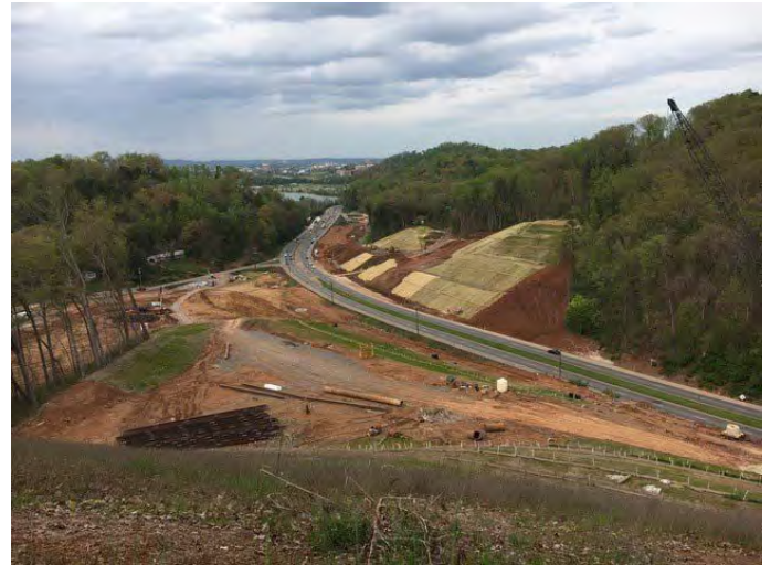
This image is during construction (April 2018) taken from the top of the hill that was deforested and relocated looking north towards the City of Knoxville at the Montlake intersection.
